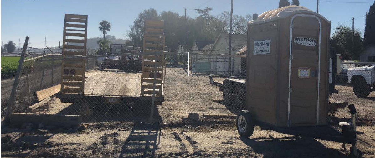
Photograph 1. (Photo point 1) View to east showing existing structures and unpaved parking area.
