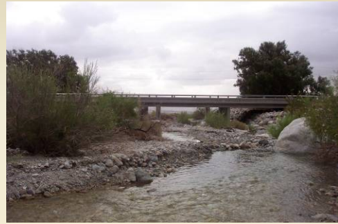
One of two bridges for Mission Creek; this is the southernmost bridge.
