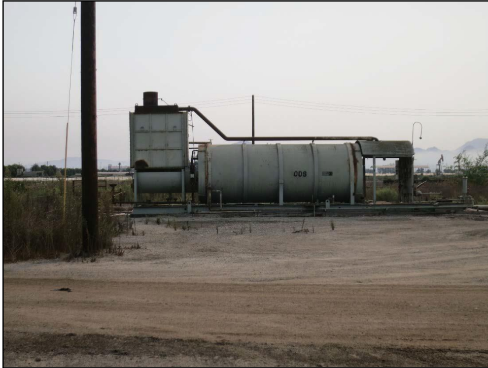
Figure 47. Detail of equipment on east side of driveway, looking east.
