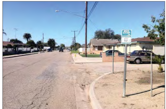
Sidewalks are discontinuous and missing from key locations such as bus stops.
