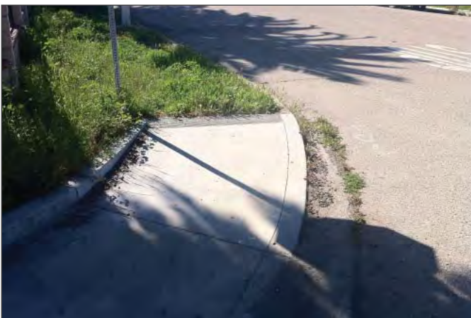
An example of one of Saticoy’s incomplete sidewalks.
