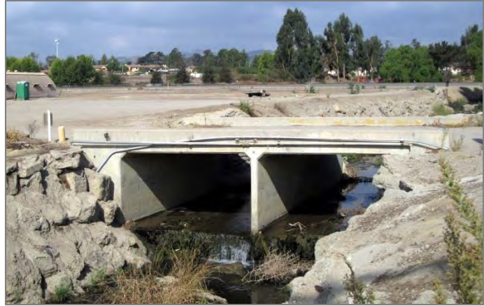
View of the existing pedestrian bridge over the Brown Barranca connecting to the unincorporated areas west of the Saticoy Plan Area
