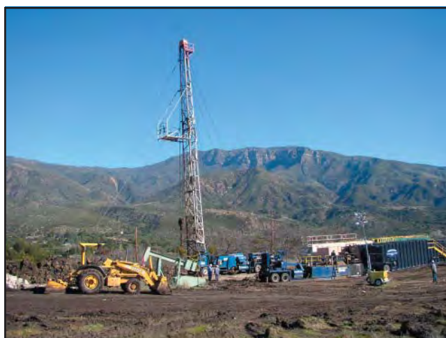
Photo 2. Key Energy Services California Inc. rig during abandonment operations on well "Ojai" 36. The Topa Topa Mountains are in the background. Photo by D. Kahler.
