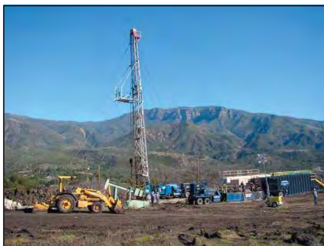
Photo 2. Key Energy Services California Inc. rig during abandonment operations on well "Ojai" 36. The Topa Topa Mountains are in the background. Photo by D. Kahler.
