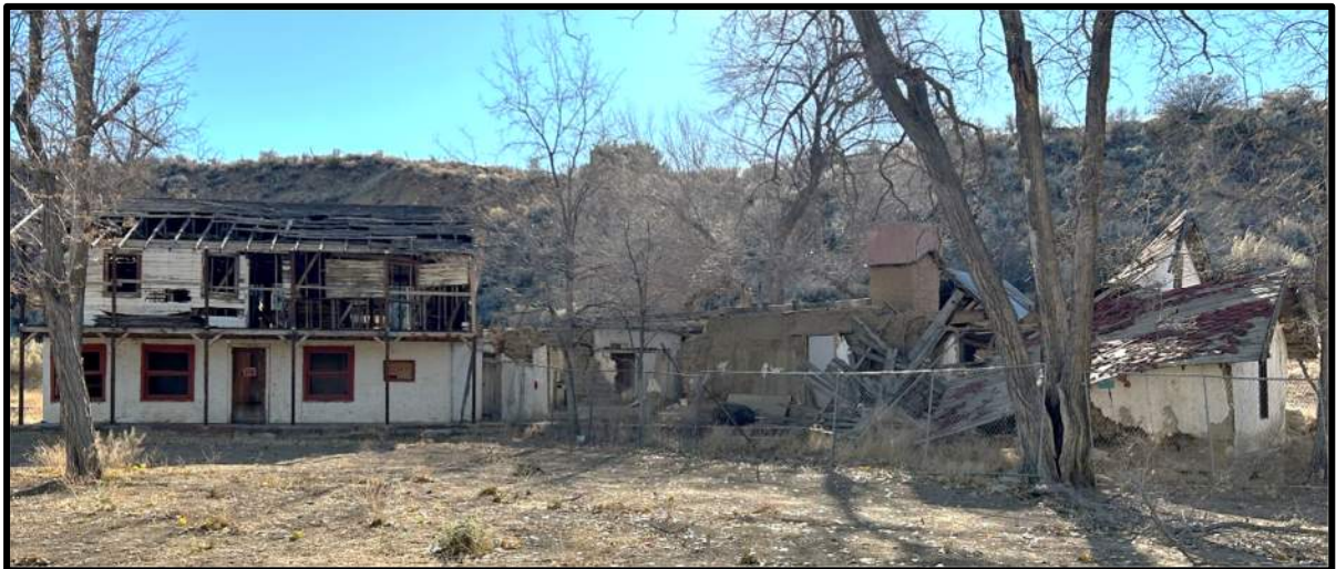
Site Photo of 1940s Addition (left) and Collapsing Adobe Buildings (right)
