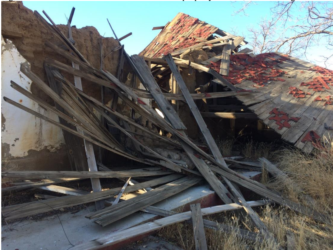
Figure 11. View showing collapsed roof and walls of northern section of the original adobe.
